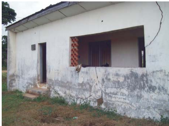
Figure 1: A Distressed Building in the Study Area Showing Cracks at the Base of the Building.
