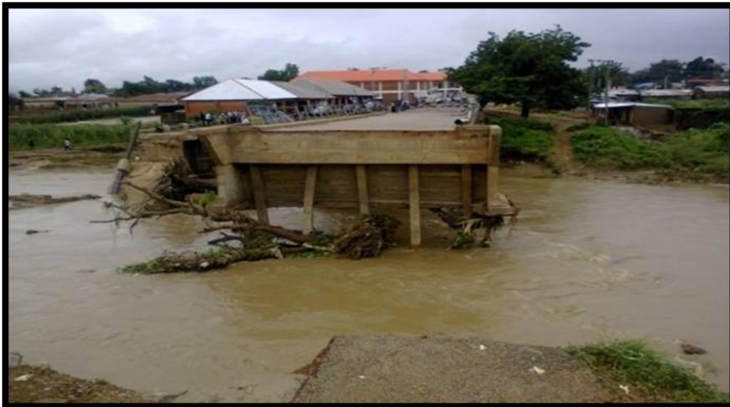
Plate 11: Collapsed Shendam Bridge. Source: (Buba Y. Alfred 2012)
